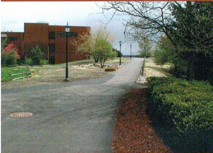
Three views from the same angle show the progress of the steam pipe and precast concrete tunnel construction project at the University of Vermont.
